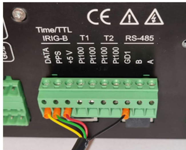
Figure 45 - Cables connected to the terminal block.
