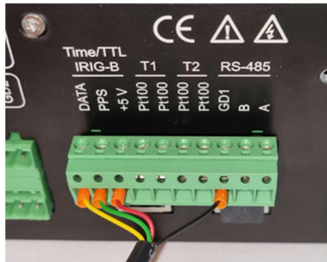
Figure 53 - Cables connected to the terminal block.
